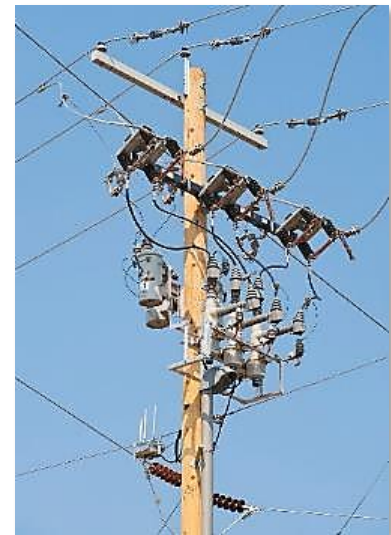
Figure 20. Dry Land Mode Device: Viper Recloser
