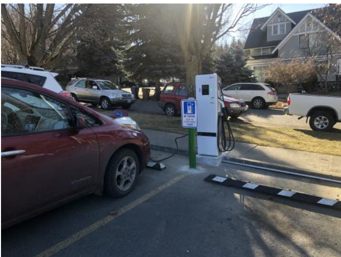
Public and workplace EVSE installed at a neighborhood shopping center (2018)
