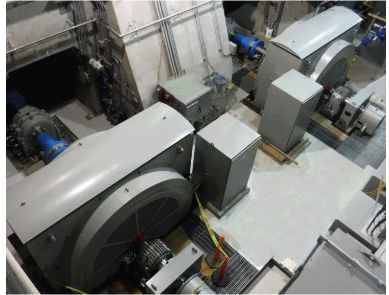
In 2016, the last two (of four) original turbine generating units at our 108-year-old Nine Mile Powerhouse were replaced with new, more efficient units as part of a multi-year project to increase the generation of clean, renewable, low-cost hydropower.
